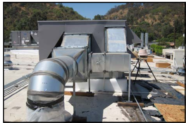
Rooftop HVAC Unit
