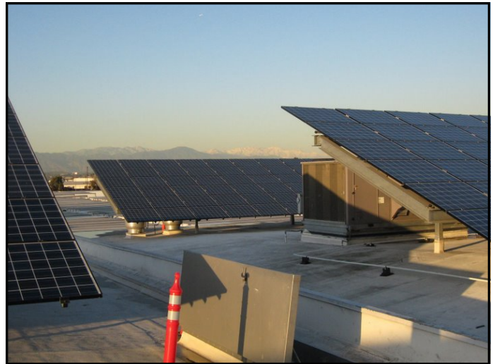
IBEW Local 11 Electrical Training Institute
